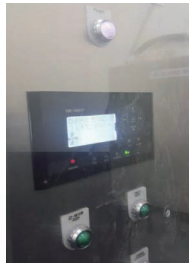
▲ Environmental Control Panel
